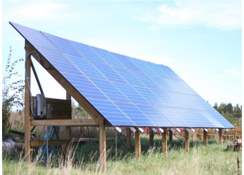
32 panel 8.64 kW Solar Array
