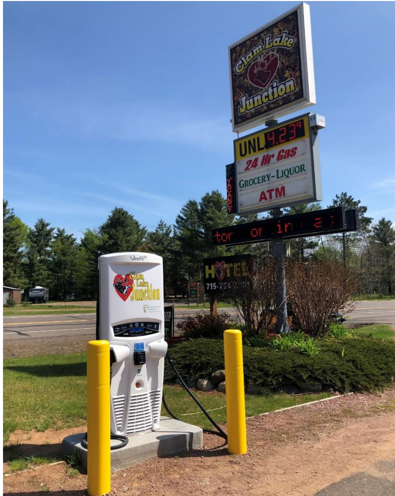
Clam Lake Junction's new EV charger
