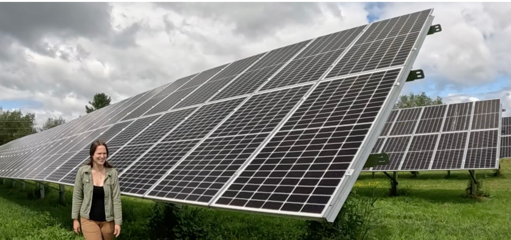
Energy Coordinator & Climate Change Specialist Jillian Wilde at Wastewater Treatment Plant microgrid
